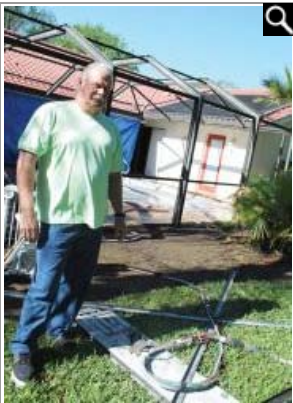
Bruce Ross restores aluminum pool cages for a fraction of the cost of replacing them.
