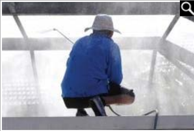
An Enclosure Rescue employee washes a pool enclosure before applying a specially formulated paint.
